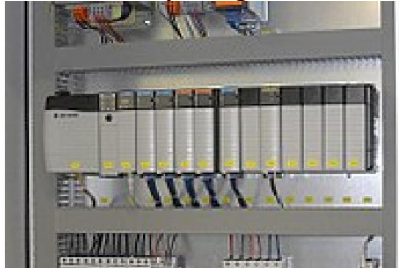
Allen-Bradley PLC installed in a control panel
